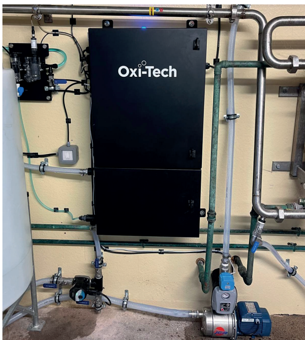
Figure 7. Pulse Oxidation System installed at Yeo Valley Farms' Yoxter Farm
